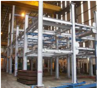
Modular Structure for Wax Plant
