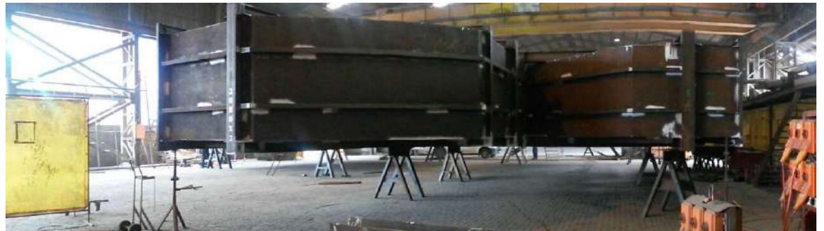
Kusile Power Station: Ducting
