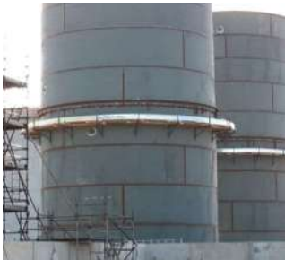
Transnet: Diversion Tanks
