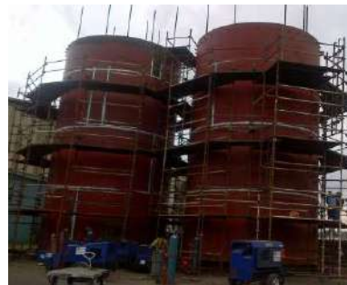
Cold Exchangers for Acid Plant
