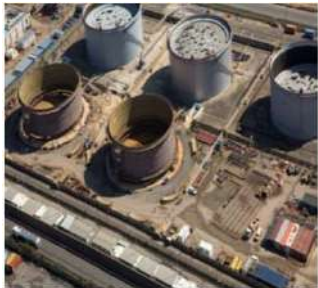
Transnet: Fuel Storage Tanks
