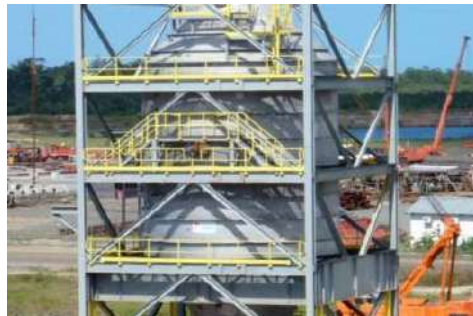
Built-in Modular Structure for Crystallisers, Nickel Mine
